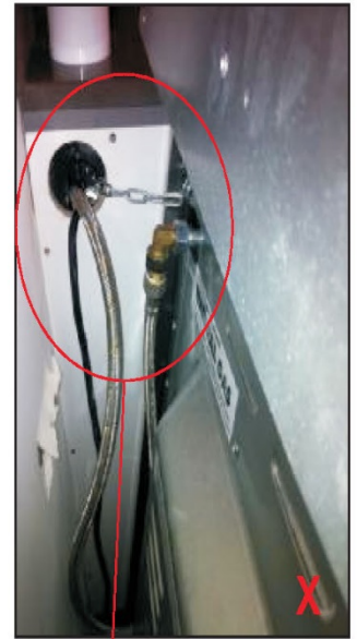
Hole in cabinet too large, allowing the upright oven to tilt forward
